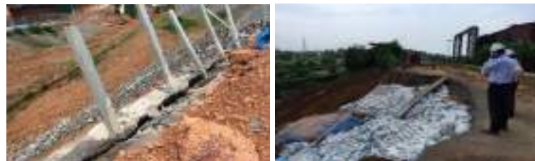
Site photographs showing extent of damage
