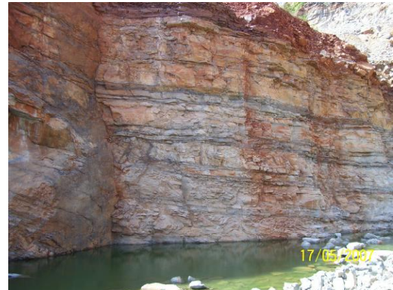
Fig. 1.1 Surface exposure of quartzite and shale at the tunnel portal, Gandikota, A.P.
