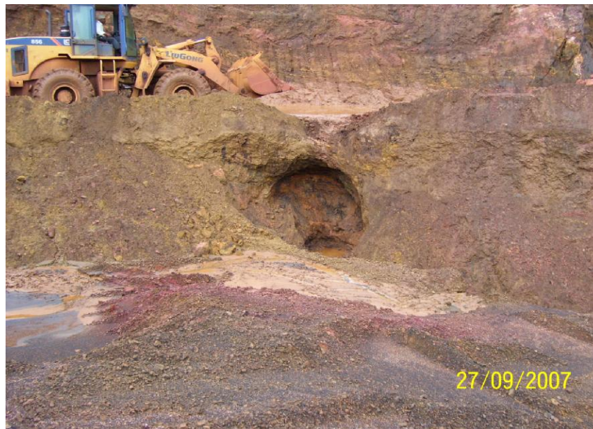
Fig. 8.4 Cavity formation in a pit slope at an iron ore mine in Goa
