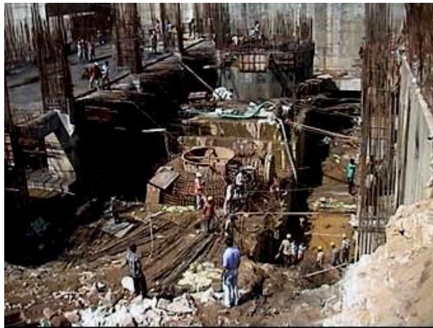
Fig. 7.3 Blasting at the proposed turbine unit 3 close to the existing turbine units 1 & 2
