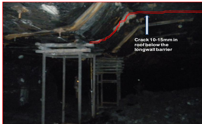
Fig. 8.4 Crack observed in CMP-3B panel below the overlying longwall barrier
