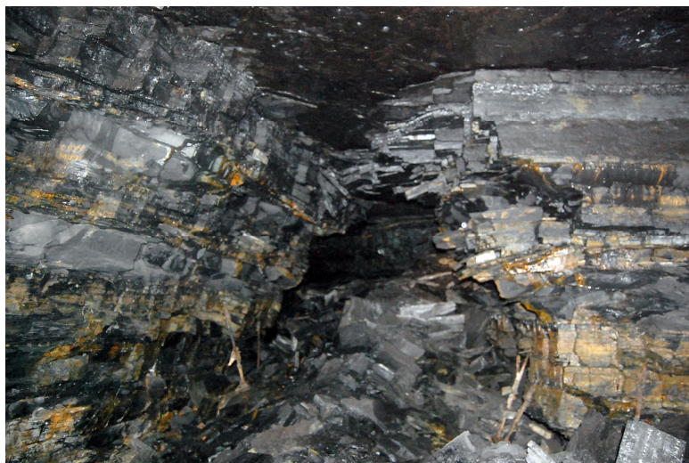
Fig. 7.2 Coal shale intercalations causing weak roof conditions at Mohan colliery
