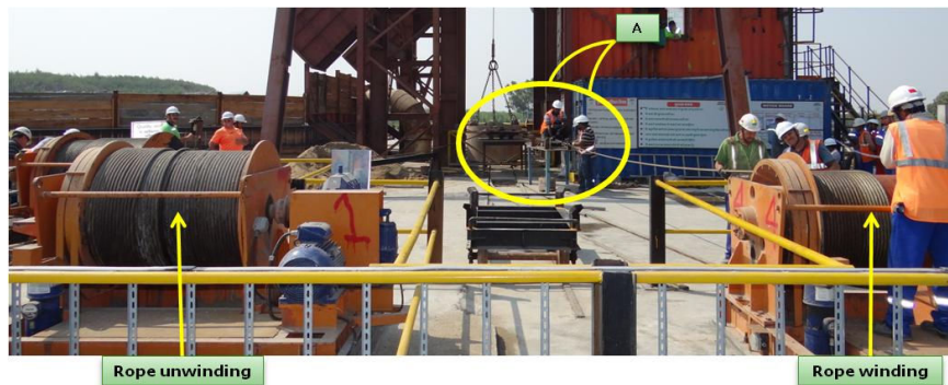
Fig. 9.2a Special arrangement made at the site for testing the winch ropes, South Ventilation Shaft
