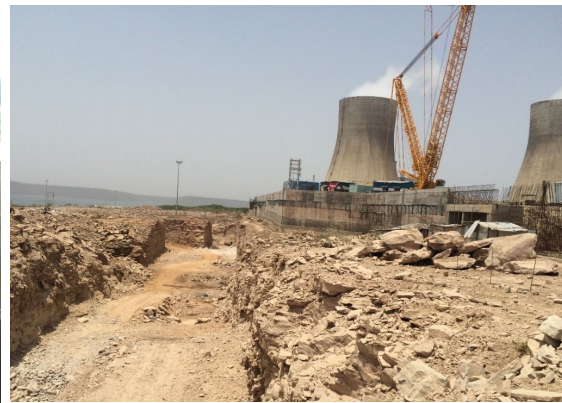
Fig. 6.4 Photograph showing the excavated cut and cover tunnel close to the retaining wall.
