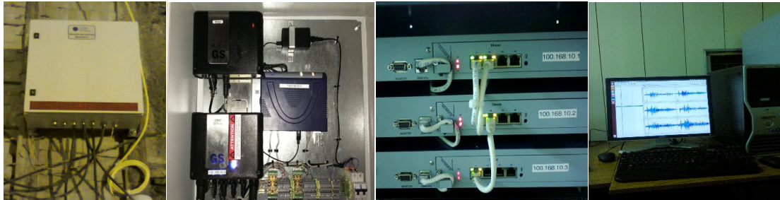
Fig. 8.2 Installed nanoseismic instrumentation at TVHPP
