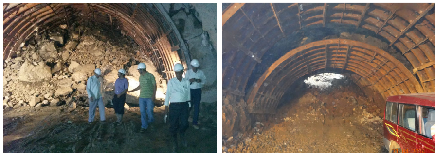
Fig. 1.3 Overbreak in left main tunnel (LMT) which was day-lighted at Ch. 3.400 km
