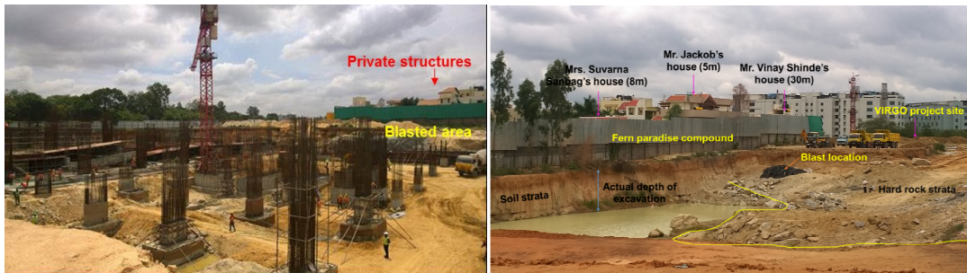
Fig. 6.7 Photograph showing post excavation & construction activity at Virgo tower area Fig. 6.8 Close in structures located on south-western side of excavation Carina area
