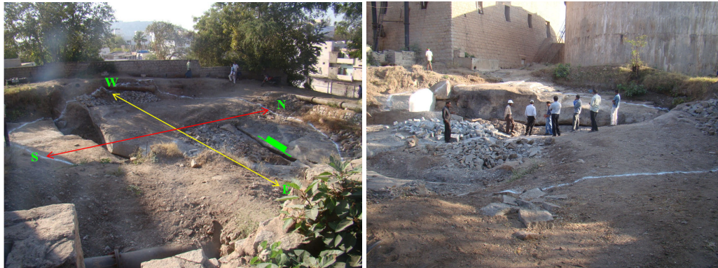
Fig. 1.8: View of foundation towards NW direction Fig. 1.9: View of foundation towards SE direction
