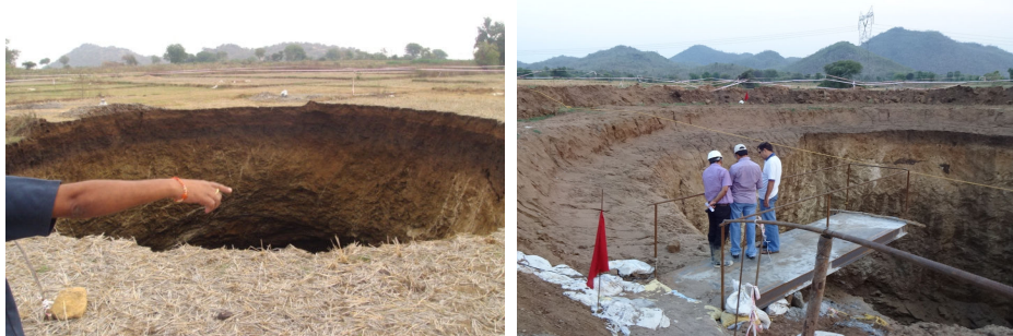
Fig. 1.4 Views of 25 m dia and 47 m deep cone shaped chimney at the surface
