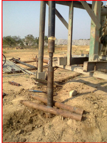
Fig. 3.2 Straddle Packer System used for Hydrofracture test at Pranahitha Chevella Sujala Sravanthi Scheme Package-12
