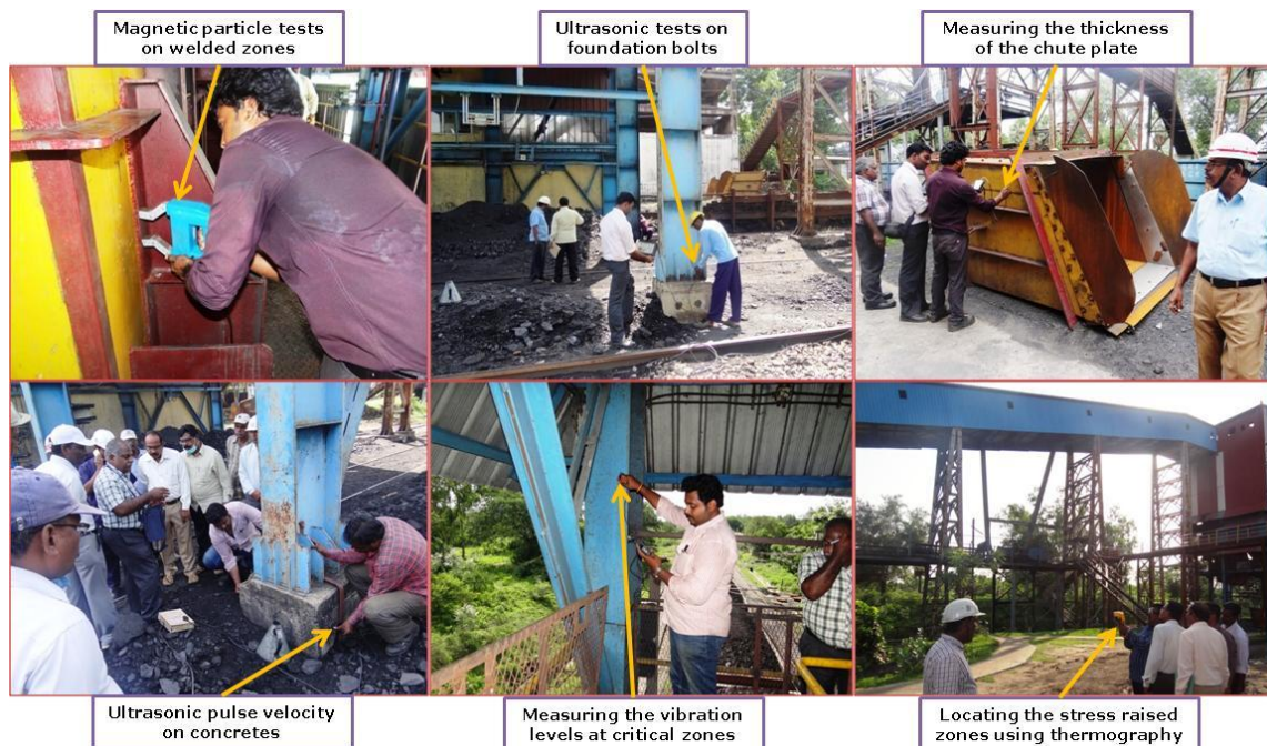
Fig. 8.7 NDT on steel structures of Ramkrishnapur Coal Handling Plant (CHP), Mandamarri Area. M/s SCCL
