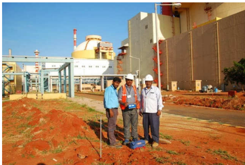
Fig. 34: Blast monitoring adjacent to reactor building 2 (Geophone buried and mike on the stand)
