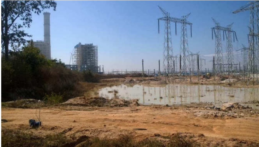
Fig. 33: Monitoring of blast vibration near switch yard area
