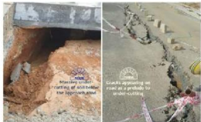
Tell-tale effect of the failure of the access road during rainy season presumably due to undercutting of soil
