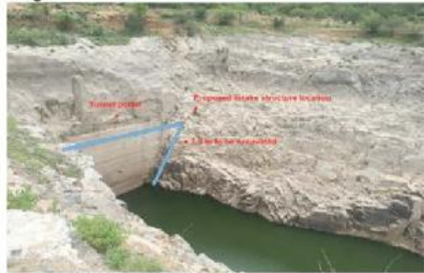
View at the tunnel portal (water level above the crown of the tunnel)
