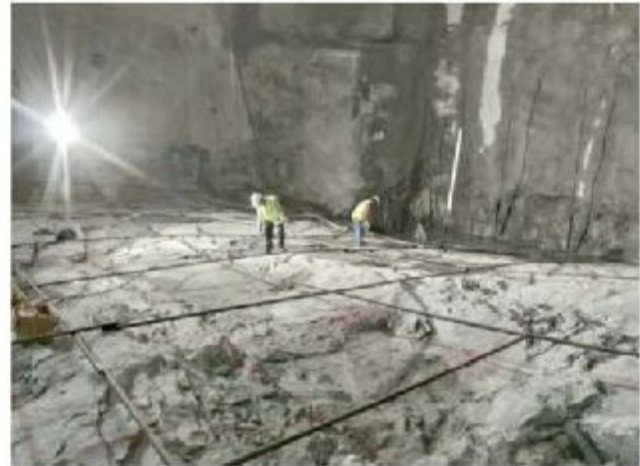
Geological mapping and collection of joint data of the foundation of pump pits
