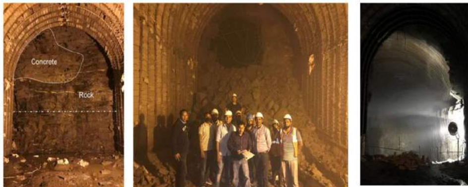
Tunnel from cable tunnel made holing through with northern wall of DSC
