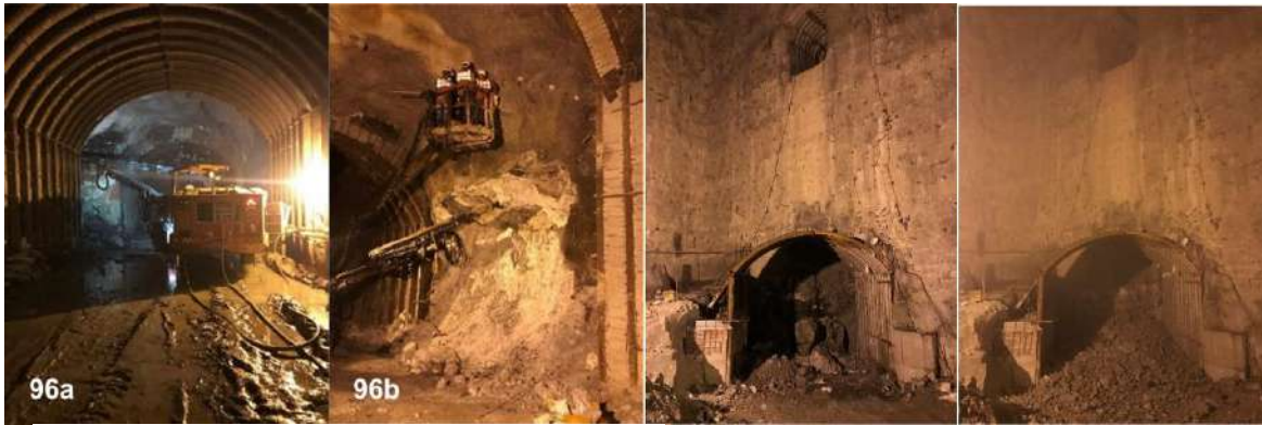
Excavation of expansion chambers at Punatsangchhu II Hydroelectric Project Pre and post blast results of Draft tube-VI excavation under critical condition
