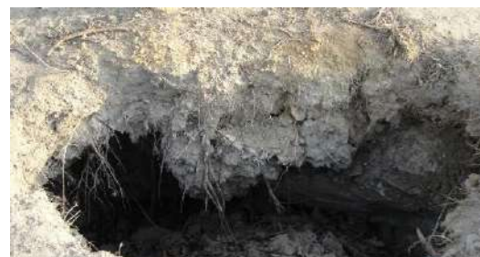
Site photographs showing damage zones to be investigated
