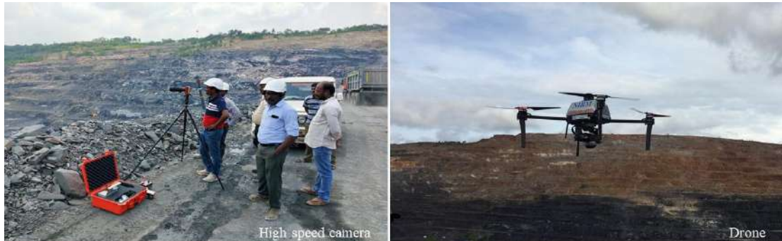
High speed camera and drone were used to optimize the blast design
