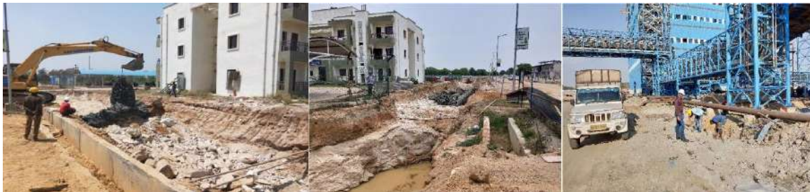
Controlled blasting near field hostel for sewerage line, close to the permanent structures of NTPC at Darlipalli STPP
