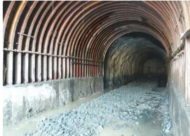
A view of completed D shape portion of pressure shaft from powerhouse
