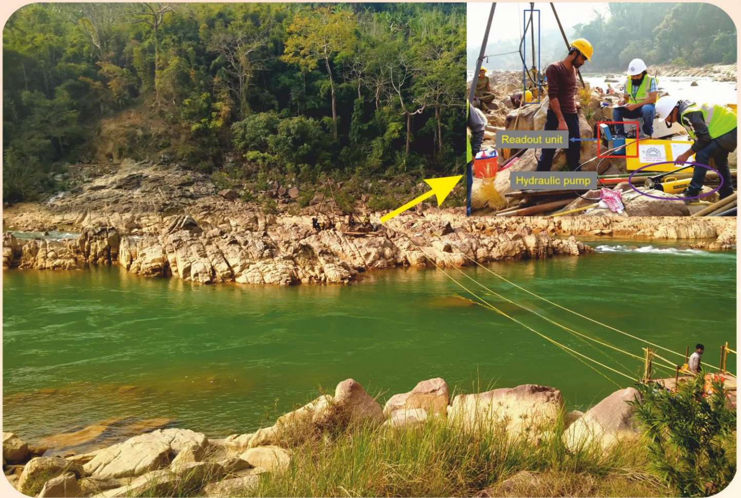
Goodman jack test conducted in a bore hole drilled at the centre of the river bed of lower Kopili hydroelectric project Assam. Inset showing the closeup view during test.
