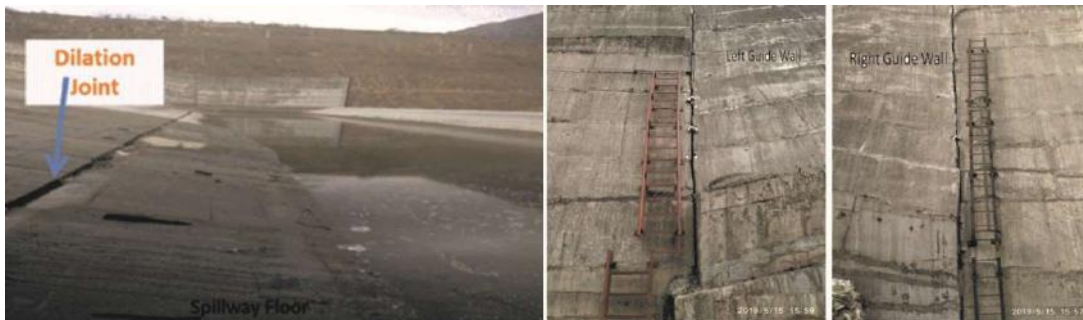
Visual damage seen around flip-bucket (left) and widening of joints on guide-wall (right)
