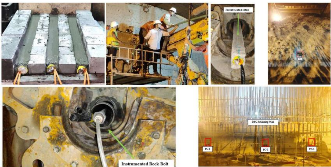
Installation of prefabricated setup comprising of load cell and biaxial borehole stress meter, Instrumented Rock Bolt in fallen muck and pressure cells to monitor lateral thrust on the retaining walls of DSC
