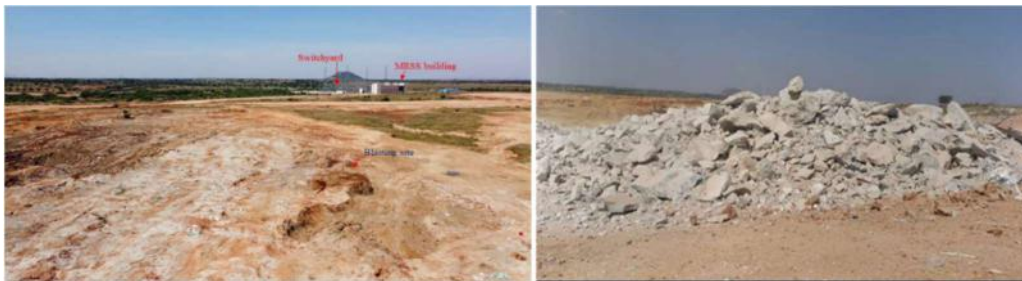
Photographs showing the structures close to blasting (left), result of post-blast (right)
