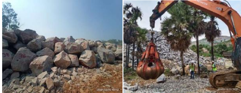
View of stock pile (left), Drop test for 1 ton armour rock (right)
