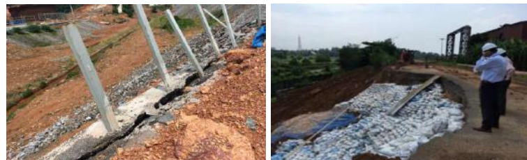
Site photographs showing extent of damage
