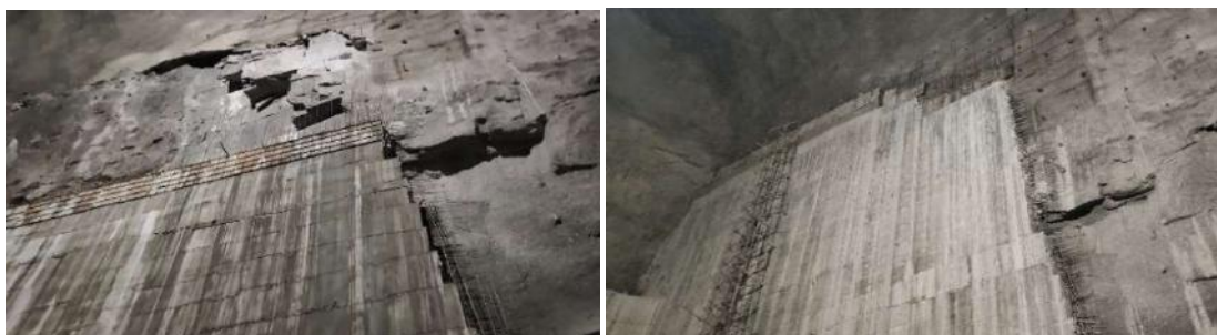
View of hanging rock blocks between EL+311.0 m and +315.0 m at D/S surge pool wall (left), View of D/S surge pool wall after treatment (right)
