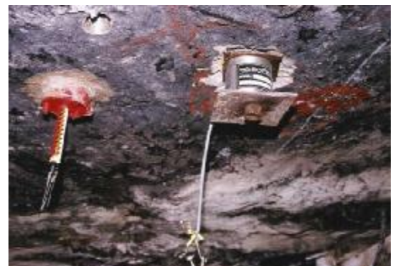
Monitoring roof behaviour in a coal mine using extensometer and load cell
