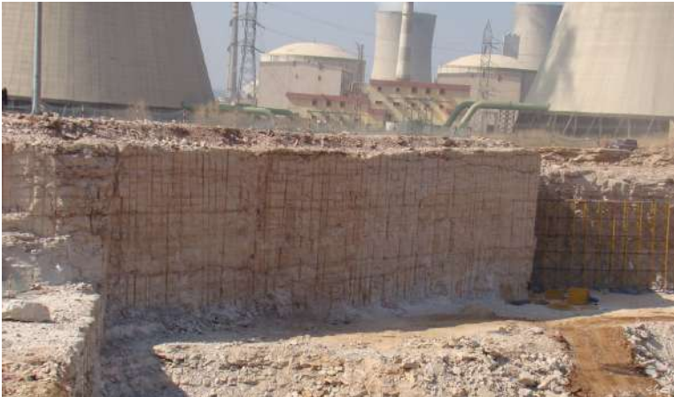
Pre-split result of 20 m high wall at nuclear power project (RAPP 7&8), Rajasthan
